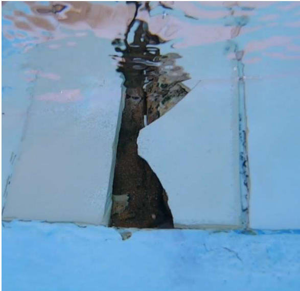
Control joint leaking – tile cracked
