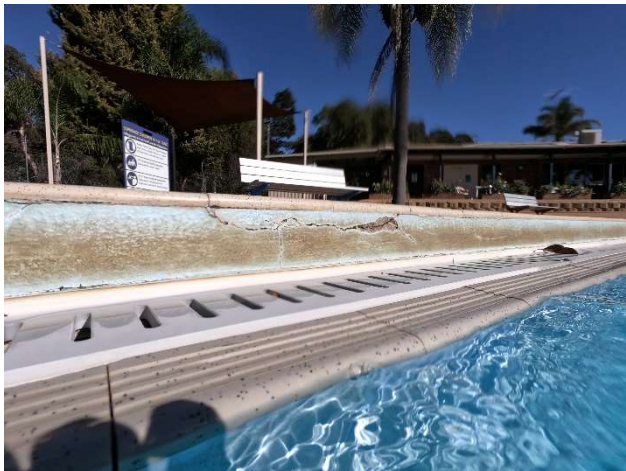
Capping screed cracking
