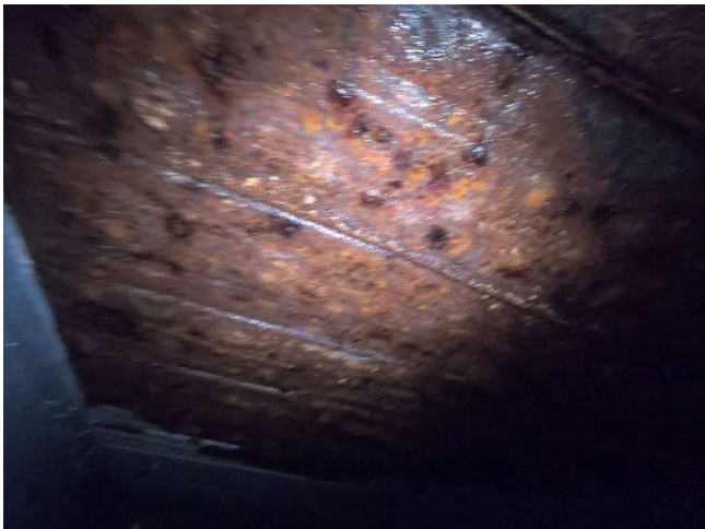
Balance tank Bondek lid rusting
