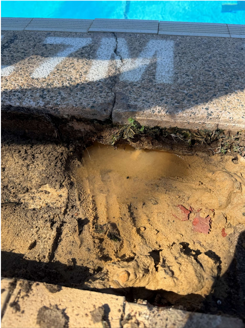
Control joint to pool leaking at dive bowl area
