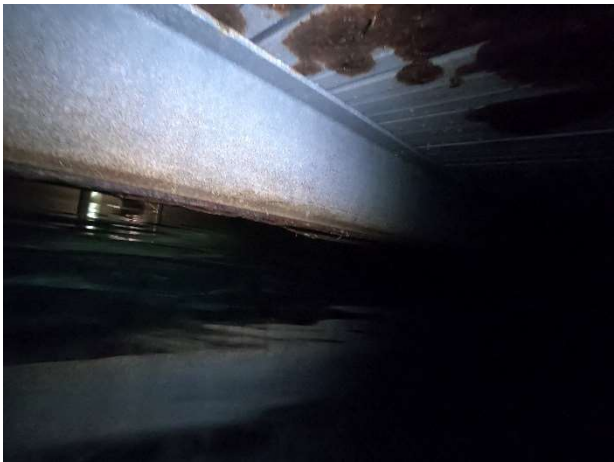
Balance tank I Beam rusting on lower section
