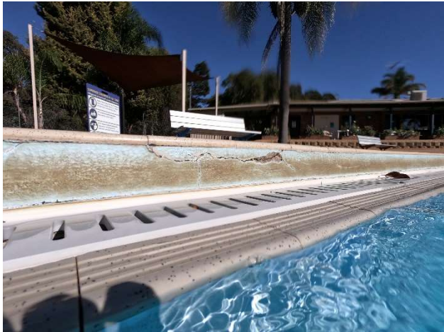
Capping screed cracking
