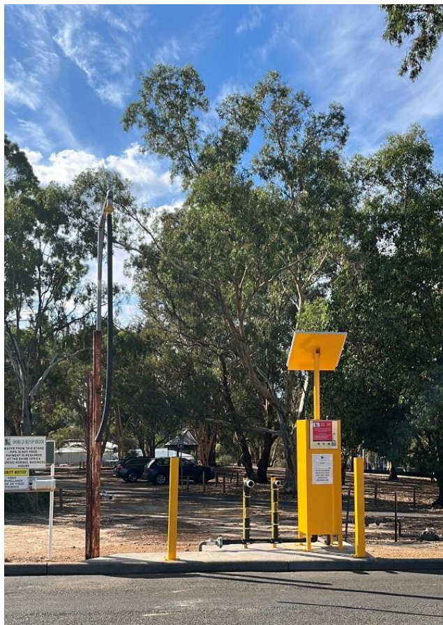
Figure 2: Swipe Card stand pipe station
