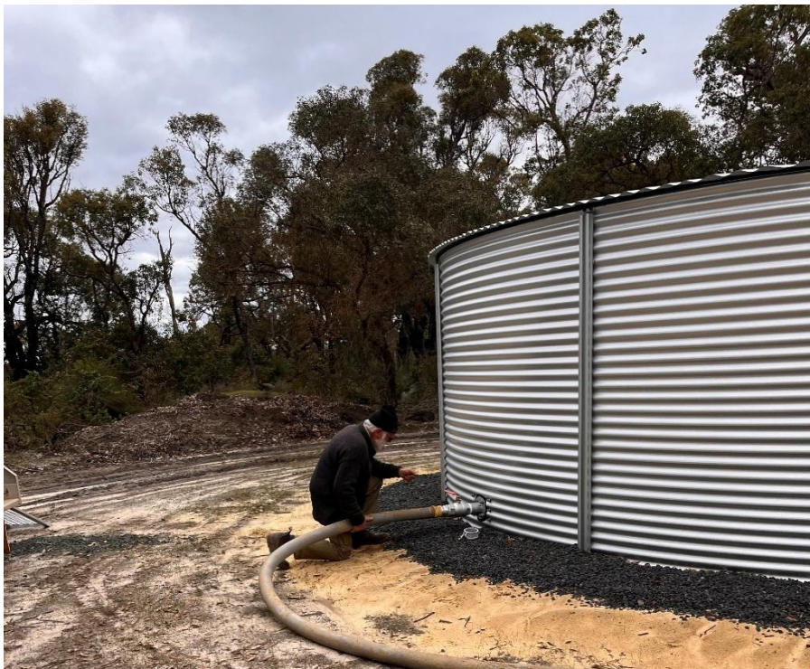
Tonebridge Fire Emergency Tank
